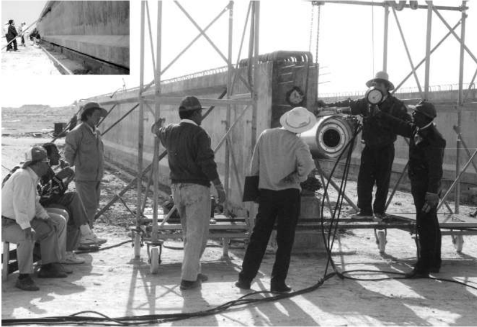
Figure 10.18 Stressing post-tensioned beam (reproduced courtesy of Hyder Consulting (UK) Ltd, copyright reserved)
