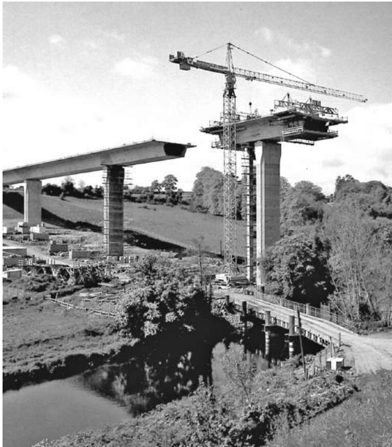
Figure 12.15 Balanced cantilever construction with bearings (reproduced courtesy of DYWIDAG-Systems International GmbH, copyright reserved)
