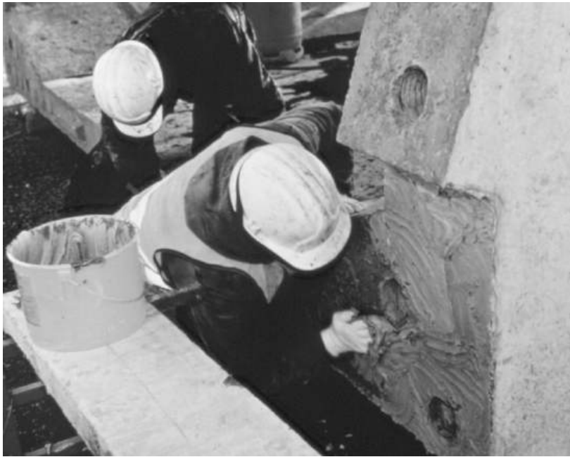
Figure 13.27 Epoxy being spread over joint (reproduced courtesy of Hyder Consulting (UK) Ltd, copyright reserved)
