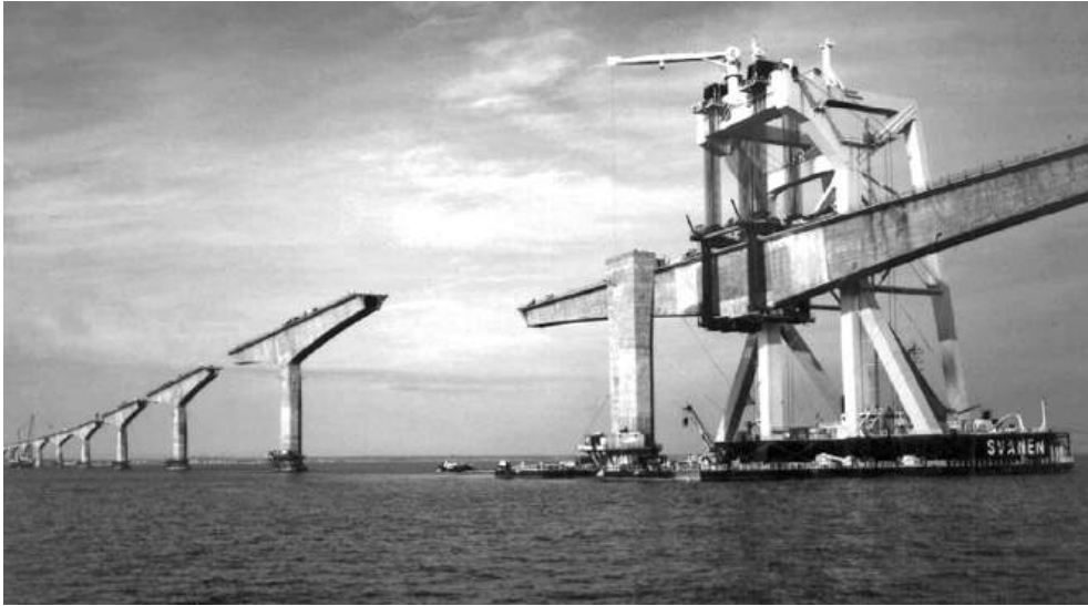
Figure 14.14 Cantilevered deck being lifted into place (reproduced courtesy of Ballast Nedam BV, copyright reserved)
