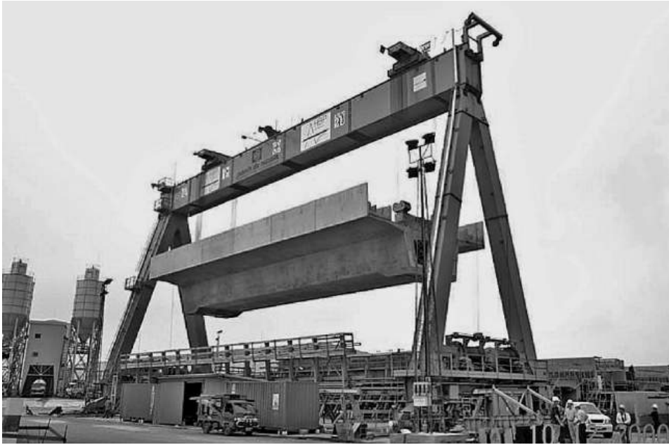
Figure 14.9 Beam with lifting gantry (reproduced courtesy of Tony Gee and Partners LLP, copyright reserved)
