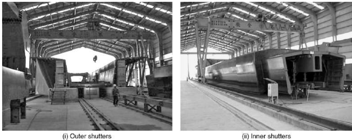
Figure 14.5 Casting cell shutters (reproduced courtesy of Hyder Consulting (UK) Ltd, copyright reserved)
