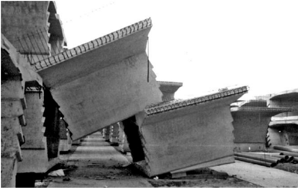
Figure 18.9 Segments toppling in storage yard
