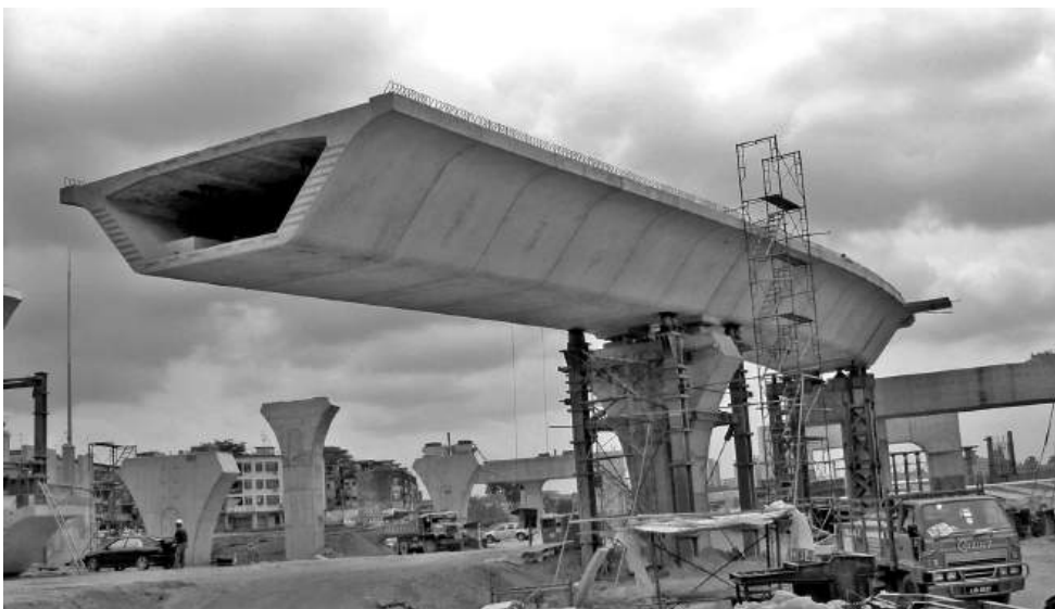
Figure 13.41 Prop and tie to stabilise cantilever (reproduced courtesy of H&T Associates, copyright reserved)
