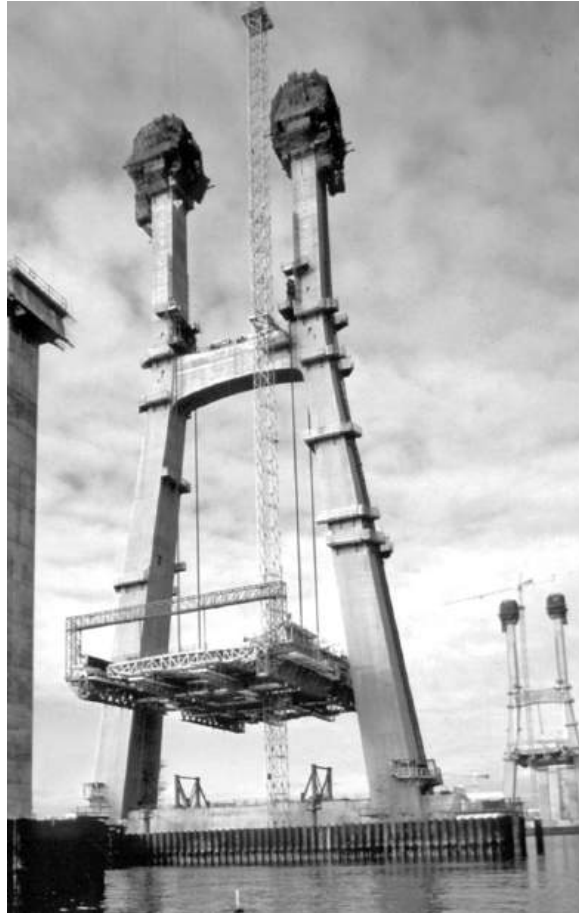
Figure 16.12 Form travellers being lifted into position (reproduced courtesy of VINCI Construction Grands Projets, copyright reserved)
