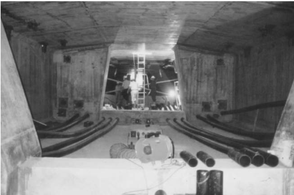
Figure 6.11 Ducts for external tendons
