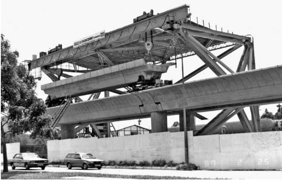
Figure 14.11 Beam being moved on to deck (reproduced courtesy of Tony Gee and Partners LLP, copyright reserved)
