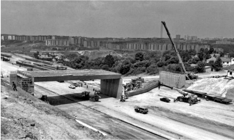
Figure 18.8 Precast beam dropped
