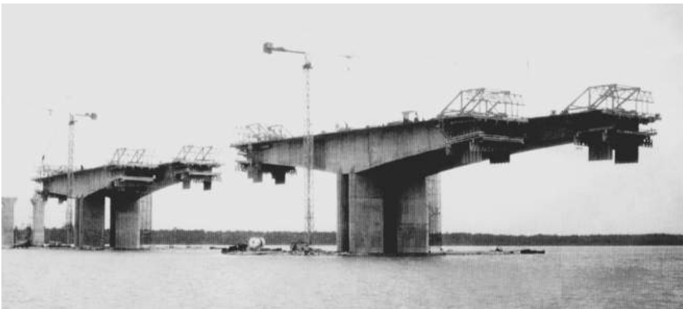
Figure 12.10 Balanced cantilever construction (reproduced courtesy of Hyder Consulting (UK) Ltd, copyright reserved)
