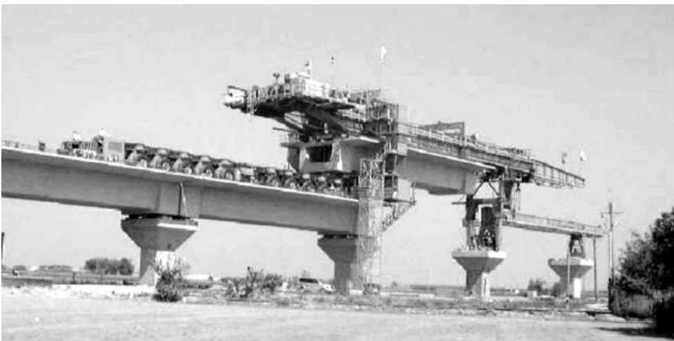
Figure 14.13 Placing beams by gantry (reproduced courtesy of Tony Gee and Partners LLP, copyright reserved)
