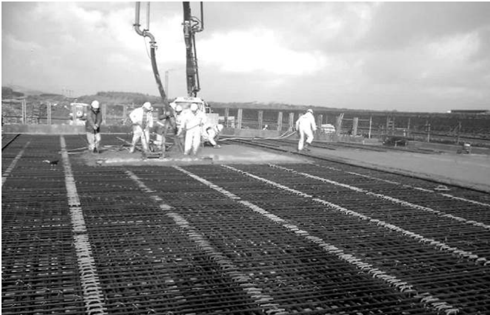
Figure 10.23 Deck slab being cast (reproduced courtesy of Hyder Consulting (UK) Ltd, copyright reserved)
