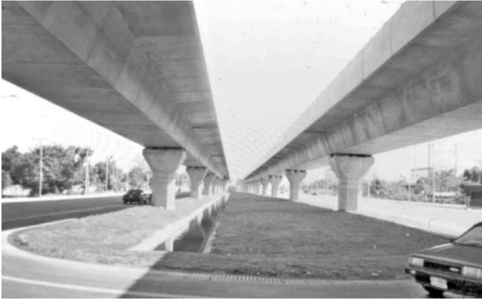
Figure 13.3 Bangkok Second Expressway, Bangkok (reproduced courtesy of Hyder Consulting (UK) Ltd, copyright reserved)
