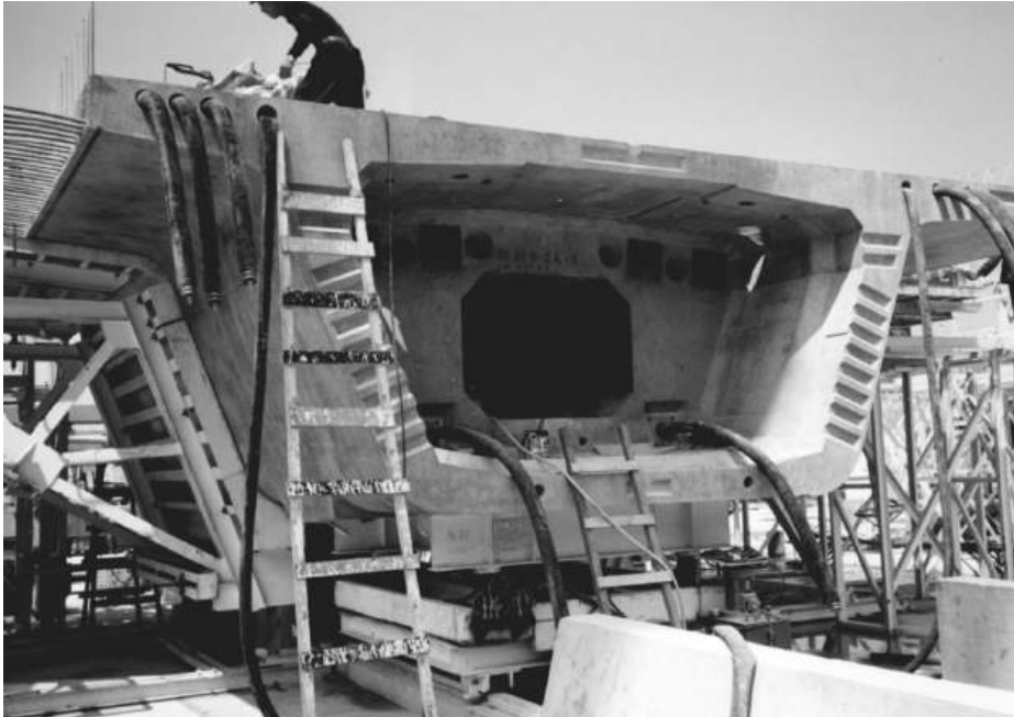
Figure 13.16 Inflated tubes in ducts during segment casting (reproduced courtesy of Hyder Consulting (UK) Ltd, copyright reserved)
