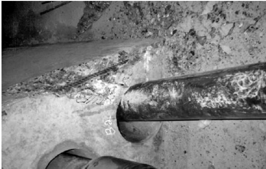
Figure 18.3 Spalling at deviator
