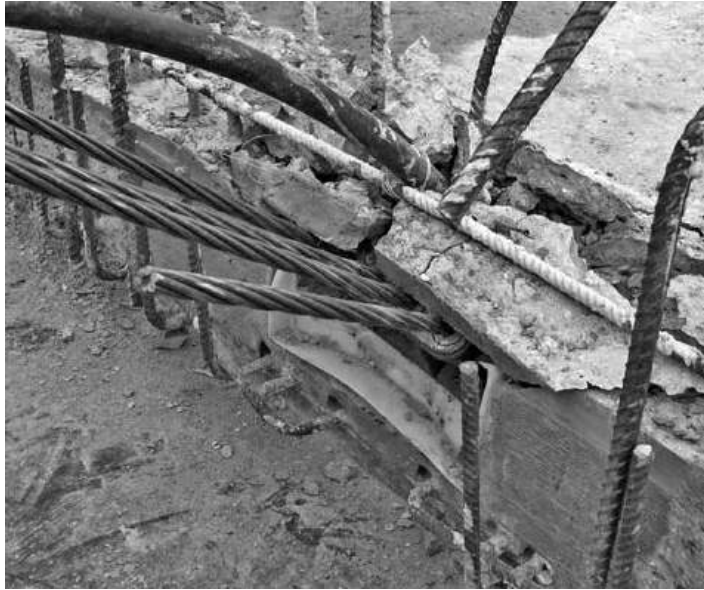
Figure 18.1 Failed transverse tendon anchor
