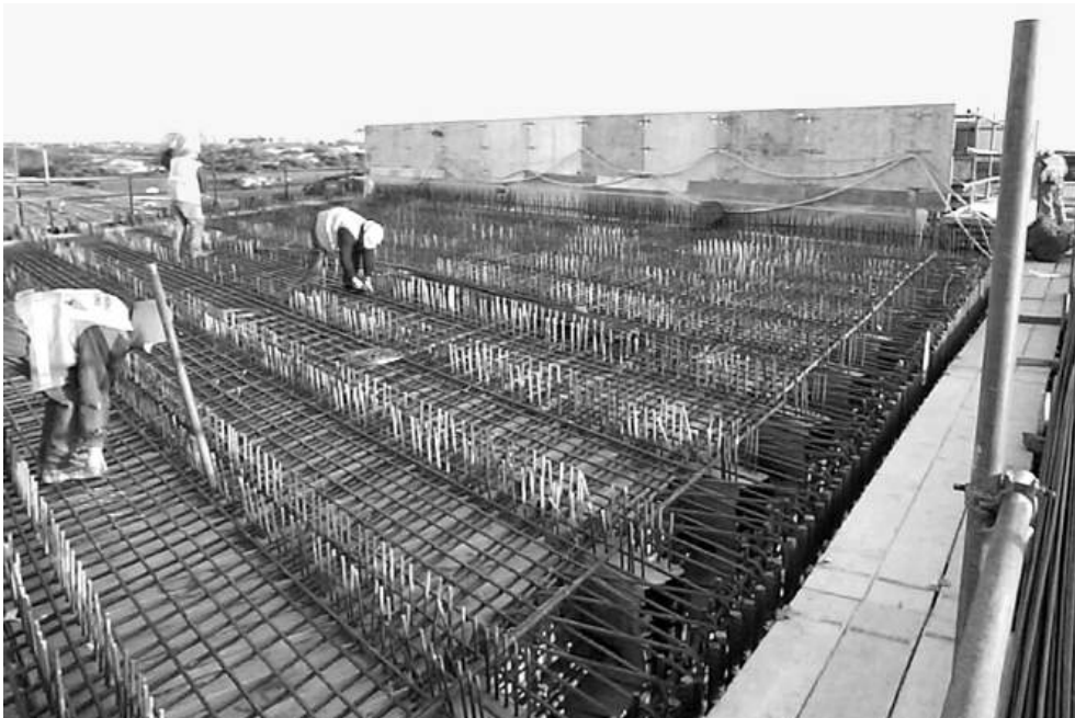
Figure 10.22 Formwork and reinforcement being placed (reproduced courtesy of Hyder Consulting (UK) Ltd, copyright reserved)
