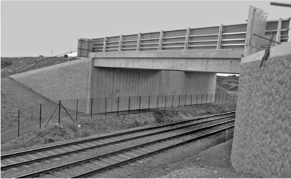
Figure 10.5 Precast beam bridge over railway (reproduced courtesy of Hyder Consulting (UK) Ltd, copyright reserved)
