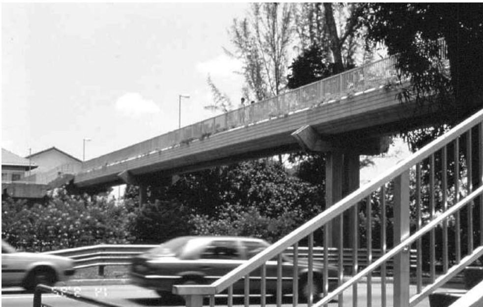
Figure 17.10 Footbridge in Singapore
