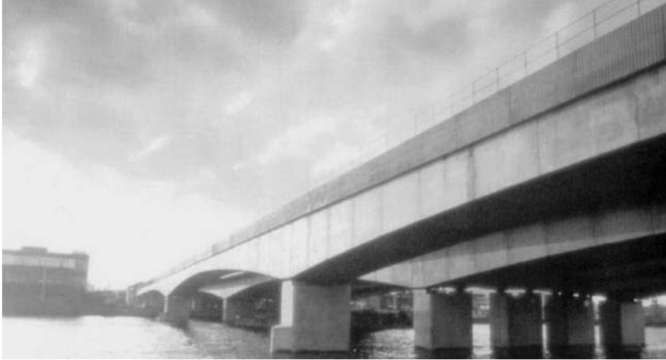
Figure 13.2 Belfast Cross-Harbour Links, Northern Ireland (reproduced courtesy of Hyder Consulting (UK) Ltd, copyright reserved)
