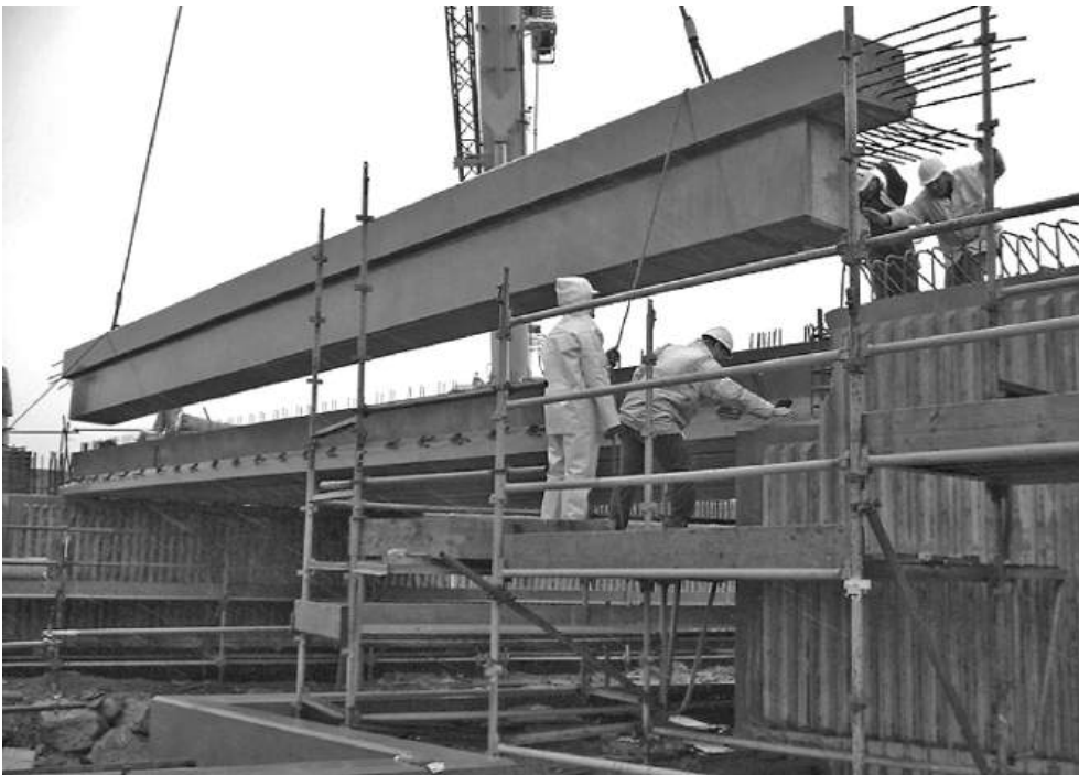
Figure 10.20 Beam placed by crane (reproduced courtesy of Hyder Consulting (UK) Ltd, copyright reserved)
