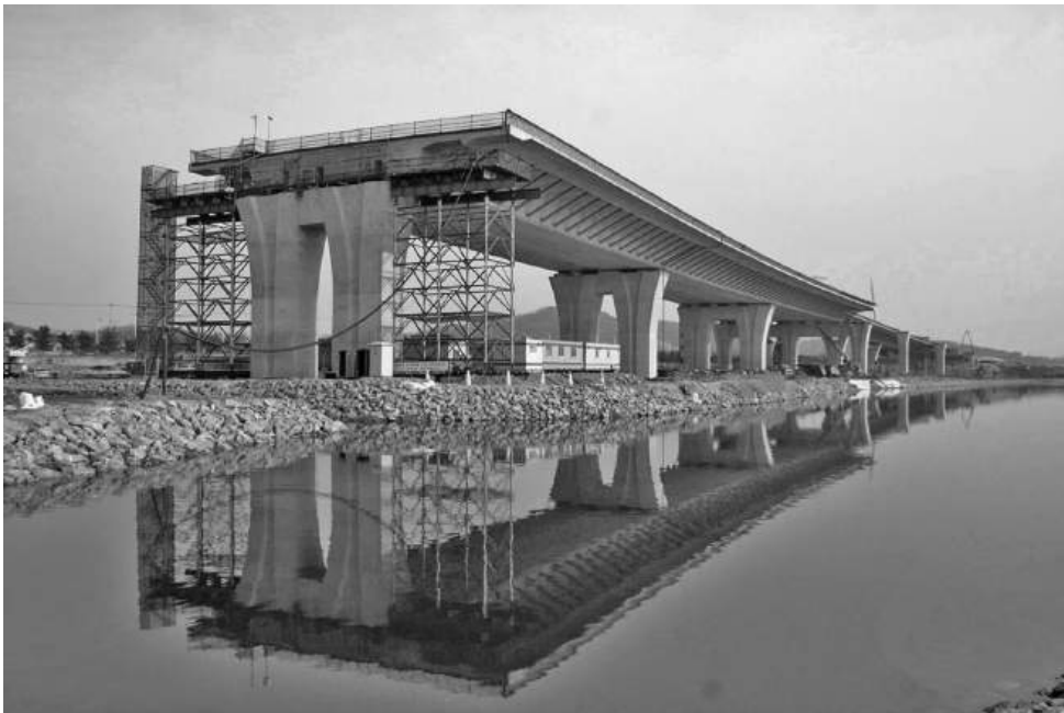
Figure 12.5 Single-cell box with struts supporting side cantilevers (reproduced courtesy of C.S. Park, copyright reserved)
