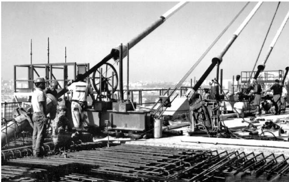
Figure 16.15 Stays being installed (reproduced courtesy of VINCI Construction Grands Projets, copyright reserved)
