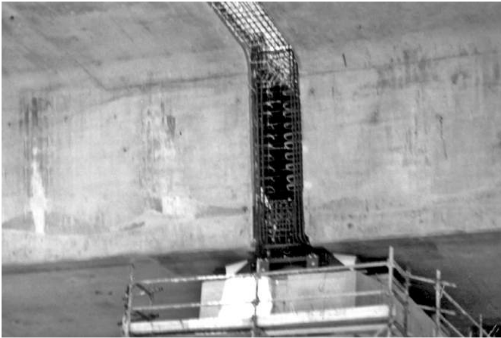
Figure 14.16 Stitch for deck continuity (reproduced courtesy of Hyder Consulting (UK) Ltd, copyright reserved)
