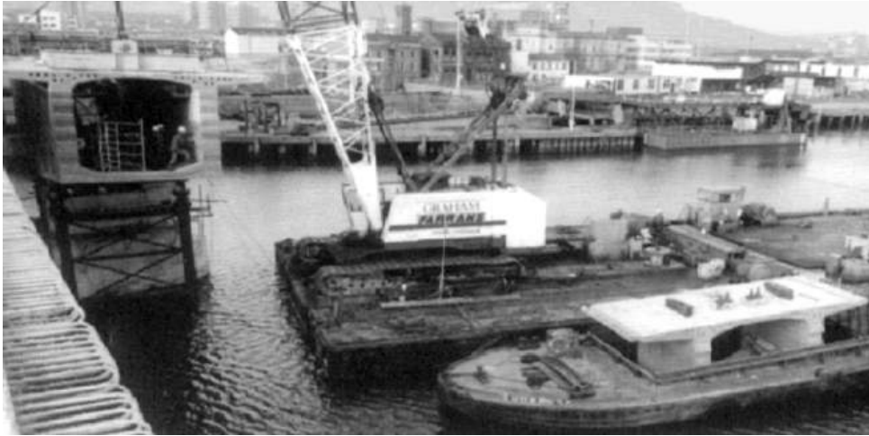
Figure 13.25 Segment transported by barge (reproduced courtesy of Hyder Consulting (UK) Ltd, copyright reserved)
