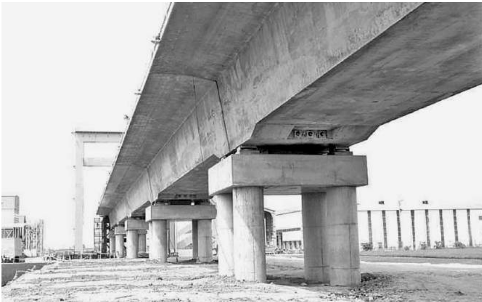
Figure 14.15 Deck on bearings (reproduced courtesy of Tony Gee and Partners LLP, copyright reserved)
