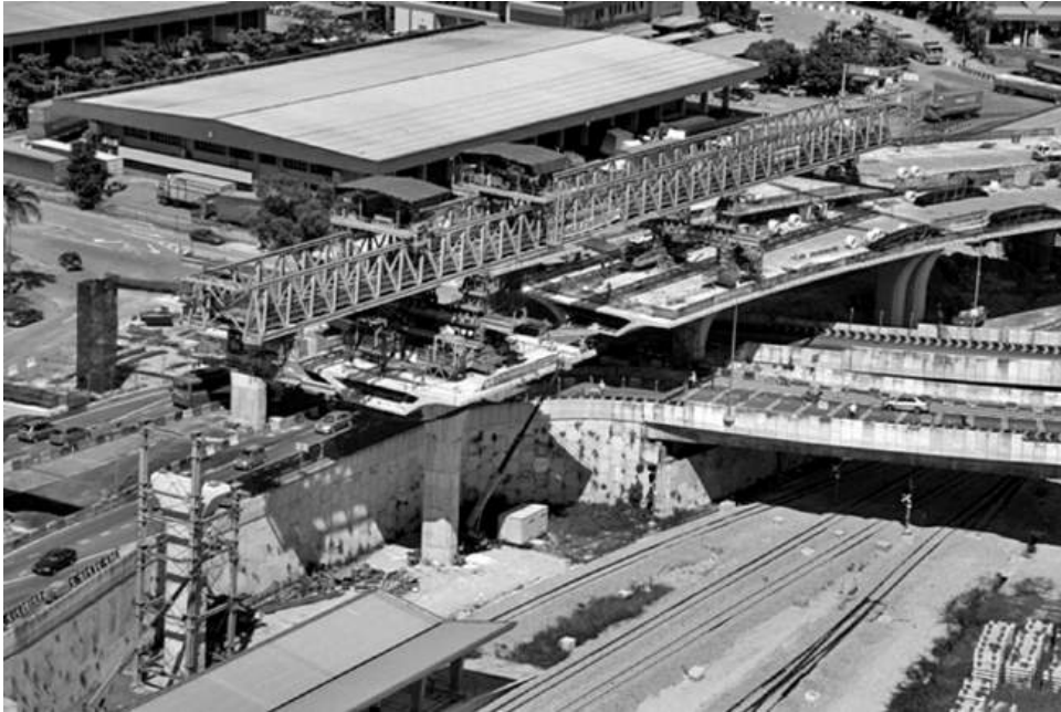
Figure 13.36 Balanced cantilever erection using a gantry (reproduced courtesy of H&T Associates, copyright reserved)
