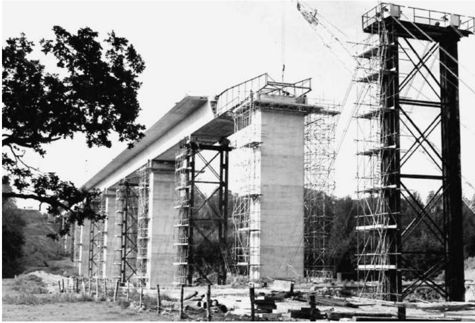
Figure 15.3 Deck during launch over piers (reproduced courtesy of Freyssinet International, copyright reserved)
