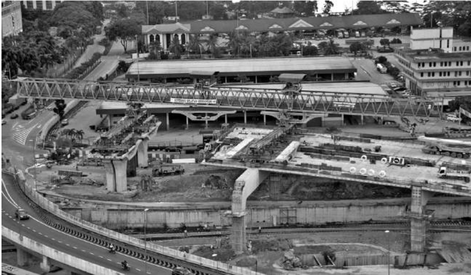
Figure 13.37 Segment being moved into position (reproduced courtesy of H&T Associates, copyright reserved)
