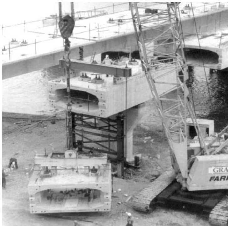
Figure 13.38 Precast segments erected by crane (reproduced courtesy of Hyder Consulting (UK) Ltd, copyright reserved)
