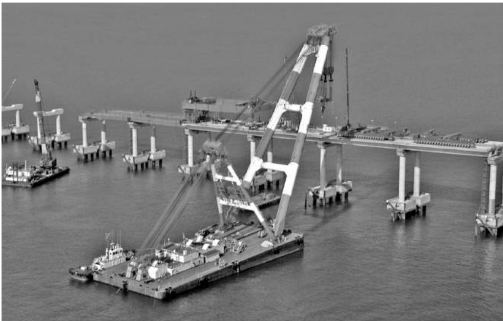
Figure 14.12 Beam being transported by barge (reproduced courtesy of Samsung C&T Corporation, copyright reserved)
