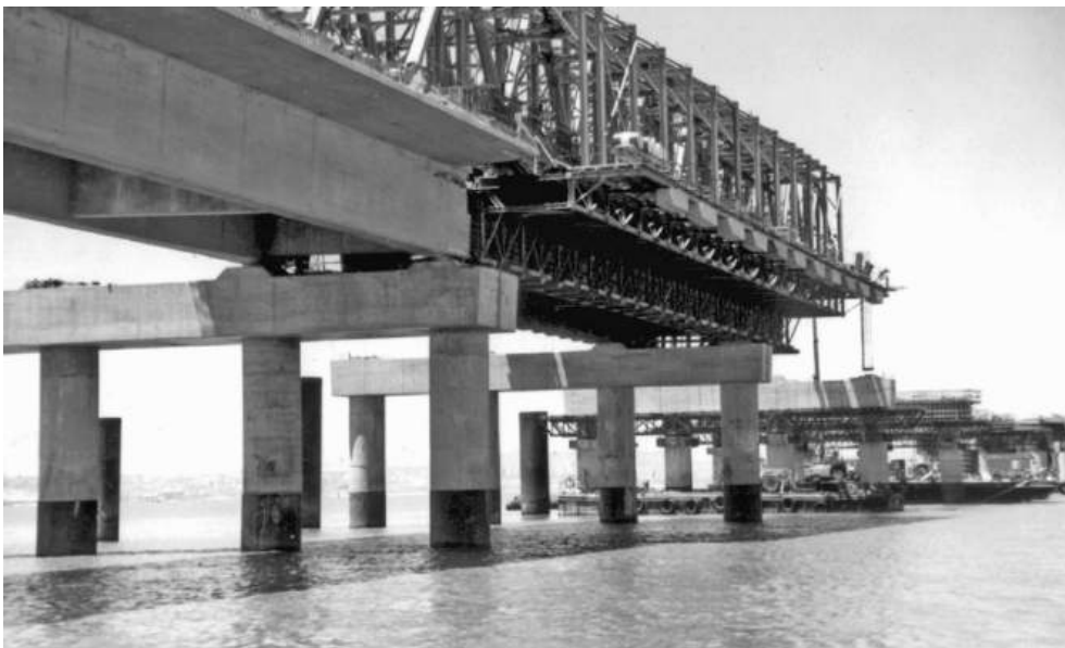
Figure 10.13 Overhead gantry for in situ beam-and-slab deck (reproduced courtesy of Hyder Consulting (UK) Ltd, copyright reserved)
